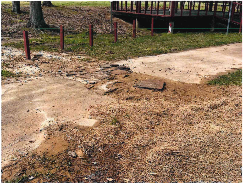
Figure 12 – City to repair broken track at Estes. Credit issued by contractor covered all locations.
