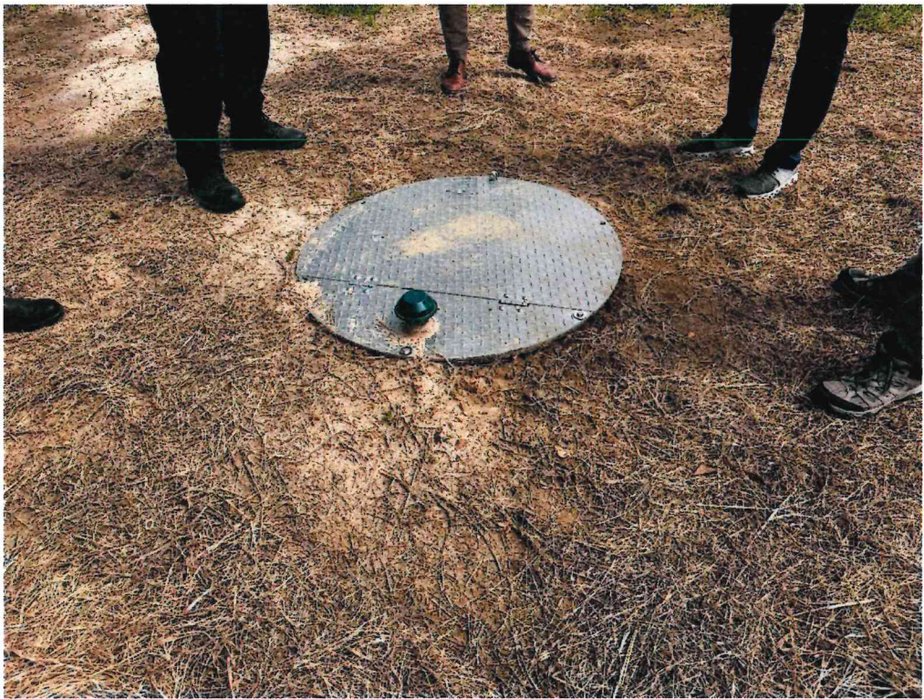
Figure 10 – Slope grade around pump cover to prevent tripping hazard.
