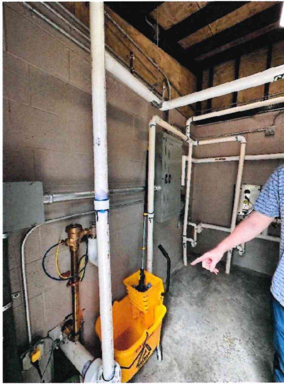
Figure 17 – Source of leak at Fairview.
