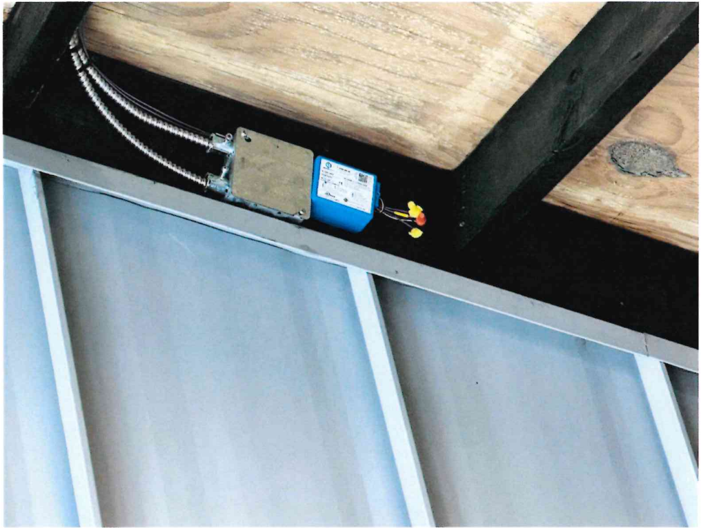
Figure 21 -Loose wires to be tucked away or hidden from guest view.
