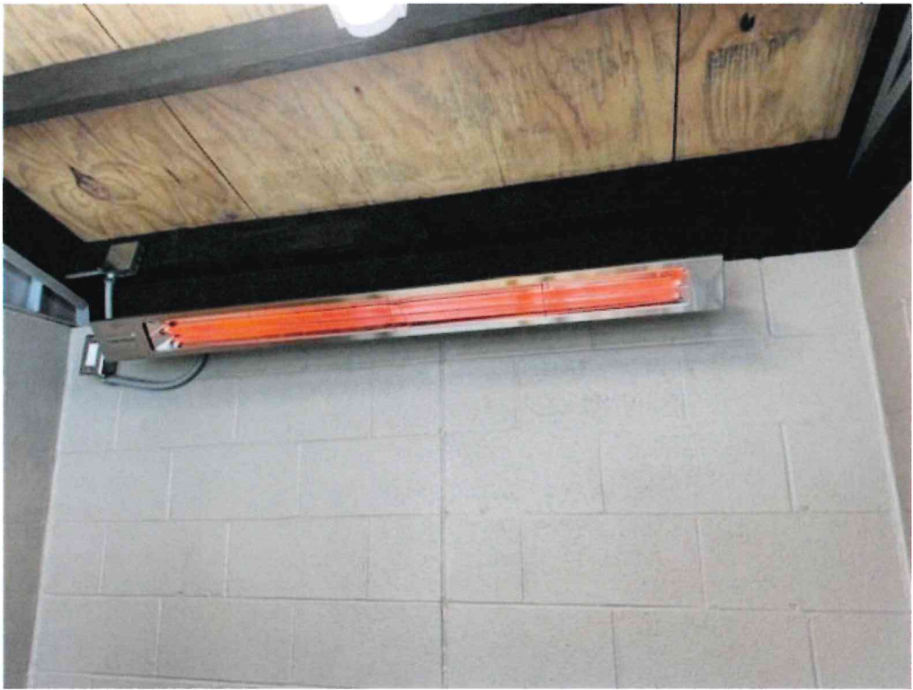
Figure 23 – Heater switches to be replaced with thermostats throughout and tamper proof cover provided. Thermostat to be relocated to neighboring wall to avoid conflict of operation.
